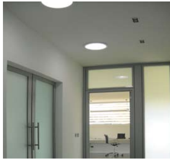
Daylighting system Almecco offices in Milan
