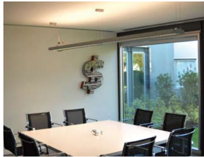
Internal lighting Almecco offices in Milan
